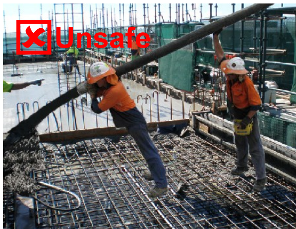
Figure 5 – Workers stretching hose for additional reach. This is an unsafe work practice.
